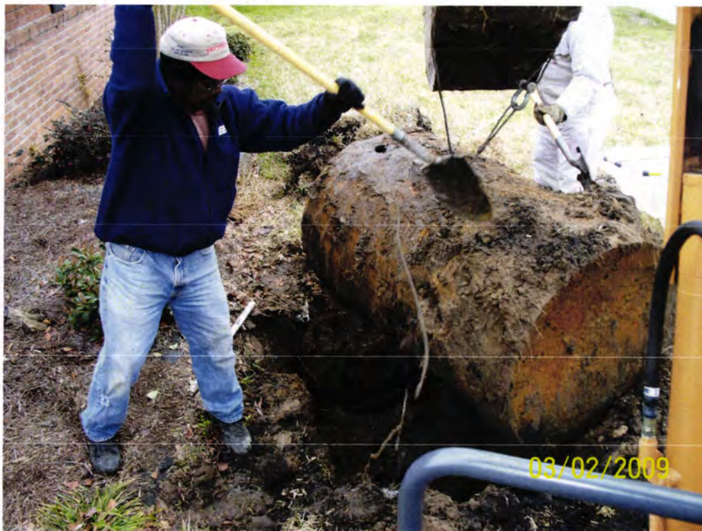
Picture 4: Loose dirt and debris being scraped off UST 120Banyan-3 immediately after removal from excavation.
